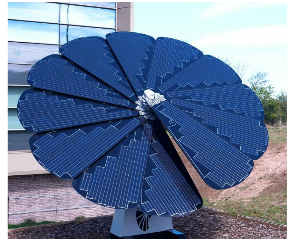
Fig. 24 - Existing solar panels installed on SEZ site.
