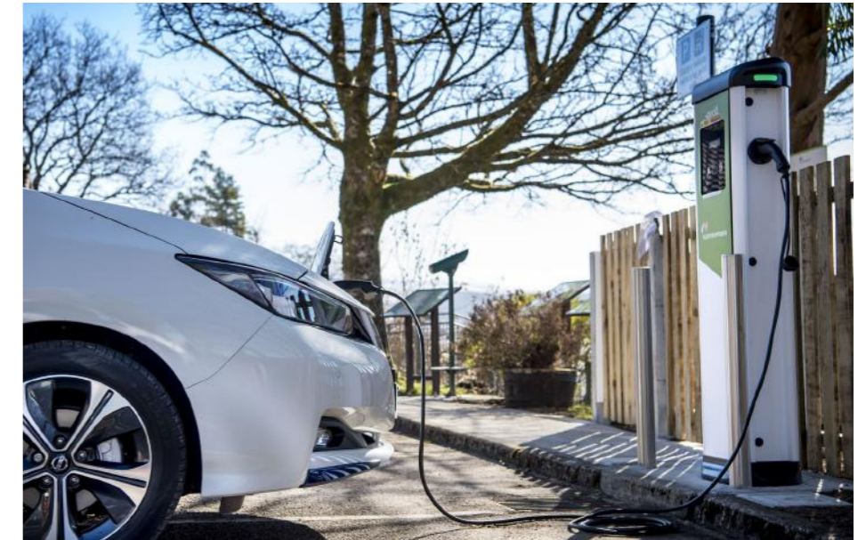
Fig. 22 - Electric vehicle charging point.
