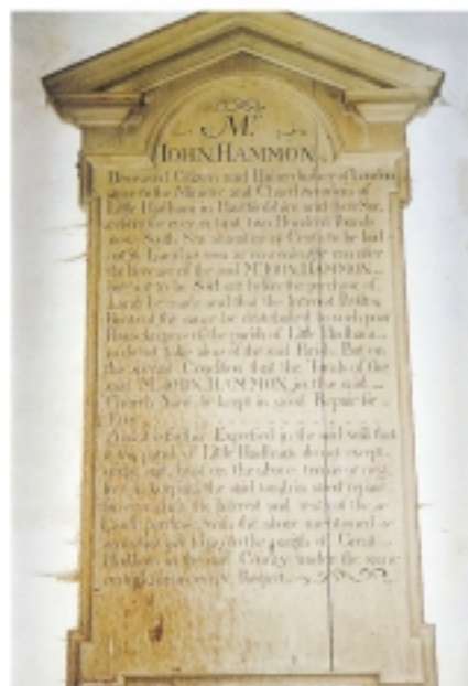
A nineteenth-century memorial board at Little Hadham Church, Hertfordshire, shows the dramatic consequences of a bat roost positioned immediately above. This concentration of excreta around the roost is typical, causing great risk to any exposed object below
