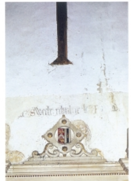
A roost site at Heydon Church, Norfolk, has been positioned above a sixteenth-century monument, which also covers part of an earlier fourteenth-century wall painting. The accumulation of bat droppings is not only visually impairing, but will also be responsible for a variety of other deterioration phenomena, both to the stonework and to the pigments of the wall painting
