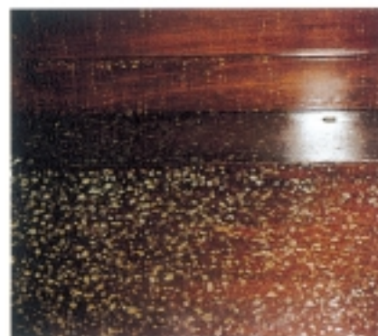
Any wooden surface previously treated with an organic varnish layer or wax coating is particularly vulnerable to the effects of bat urine. Here the polished top to an organ at Clayton Church, East Sussex, displays the typical effects of surface etching resulting from the strong alkalinity of bat urine when in contact with such coatings
